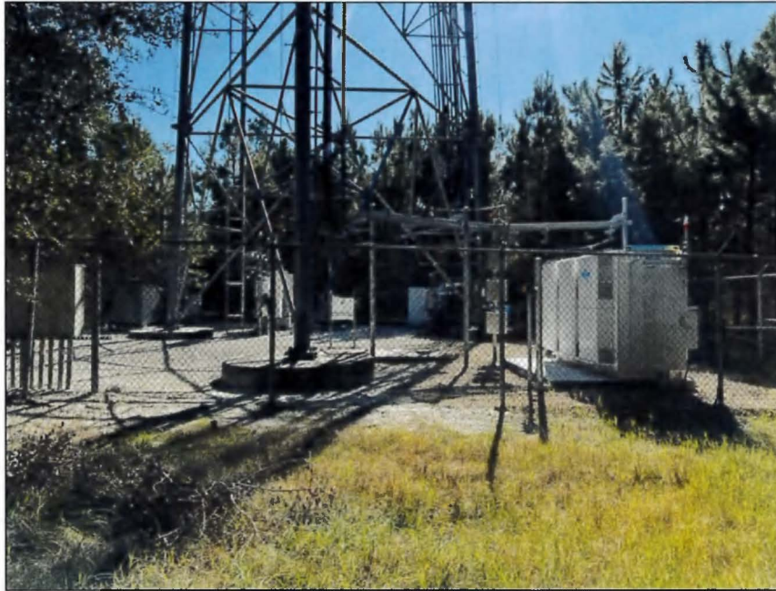
3 - Photo 3 Cell tower
